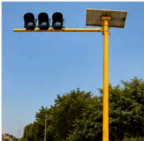
05 TRAFFIC LIGHT POLE PROJECT
